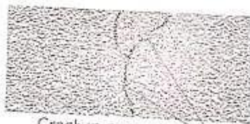
Crack in concrete due to shrinkage
