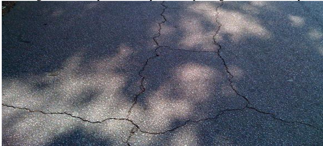
Fig. Block Cracking
