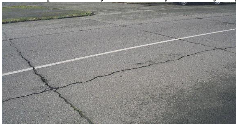
Fig. Joint Reflection Cracks
