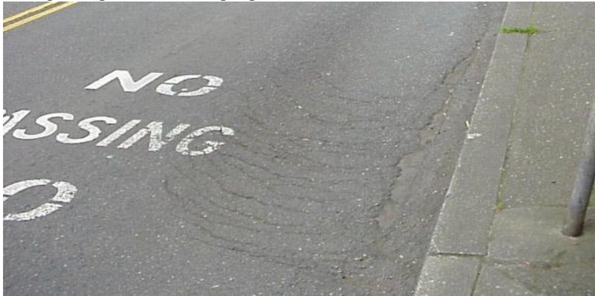
Fig. Slippage Cracks
