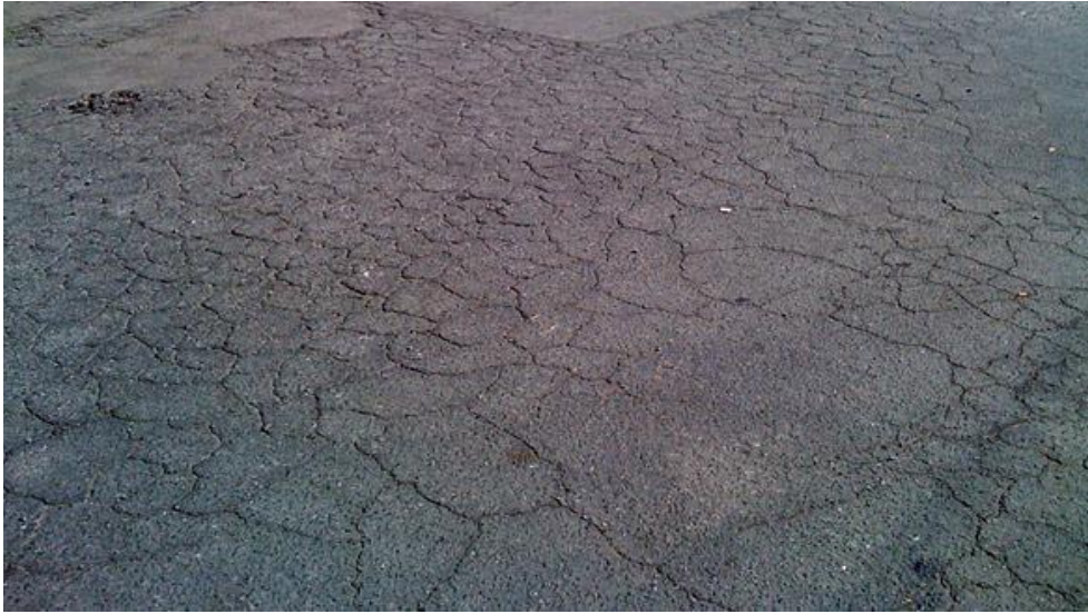
Fig. Alligator Cracking
