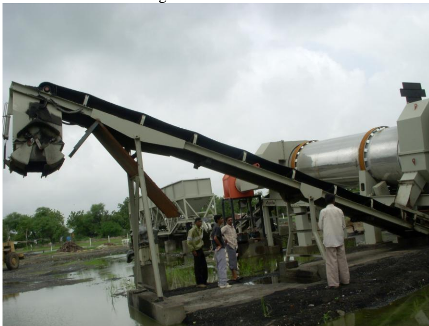
Fig. Load Out Conveyor
